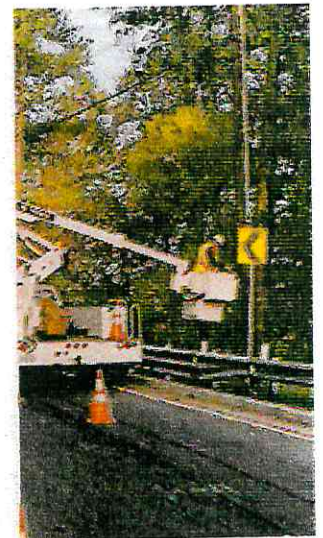
Electric & Existing Pole
