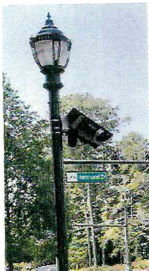
Solar & Existing Pole
